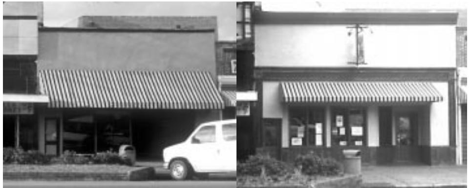
Renovation work to the c. 1900 building for the Milledgeville Locos included stucco repair, a new wood framed storefront, and wood trim sign banding.
